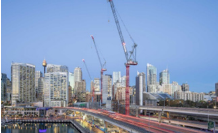
3. Figure – The Construction of The Ribbon (a hotel, apartment building, retail store and movie theatre ) in Darling Harbor Sydney, Australia.
