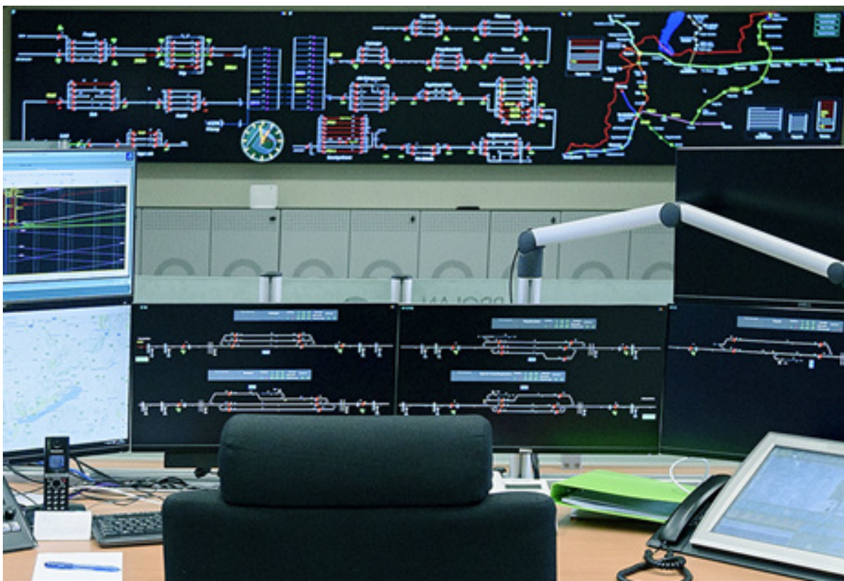
1. Figure - Prolan work station
